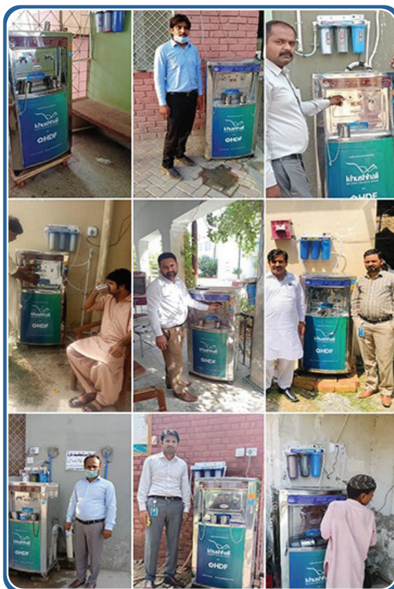
Water Coolers with Filters Installed across Pakistan
